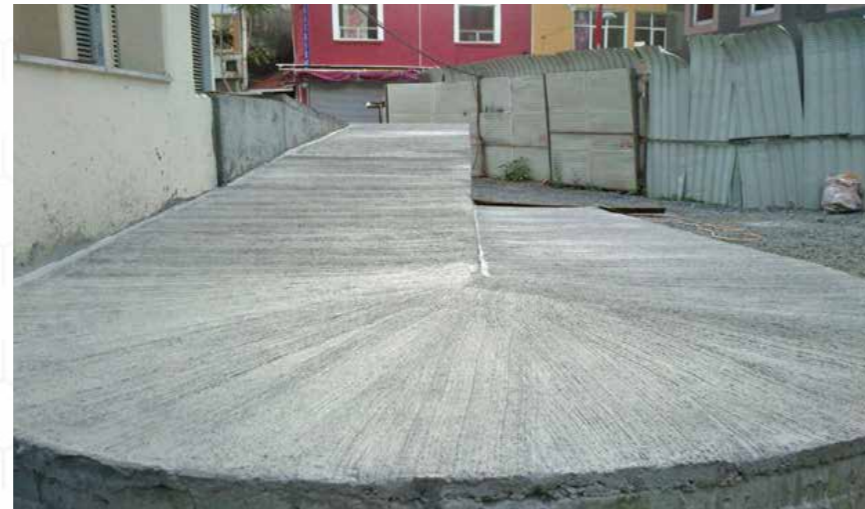
Construction of Infrastructure for West and East Ventilation Shaft & Sarayburnu storage site. Construction of Compacted Back II, RC Ramps and Stairs at West and East Ventilation Shaft.
